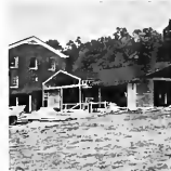
The scene behind Talge Hall as the new dean's house goes up.
