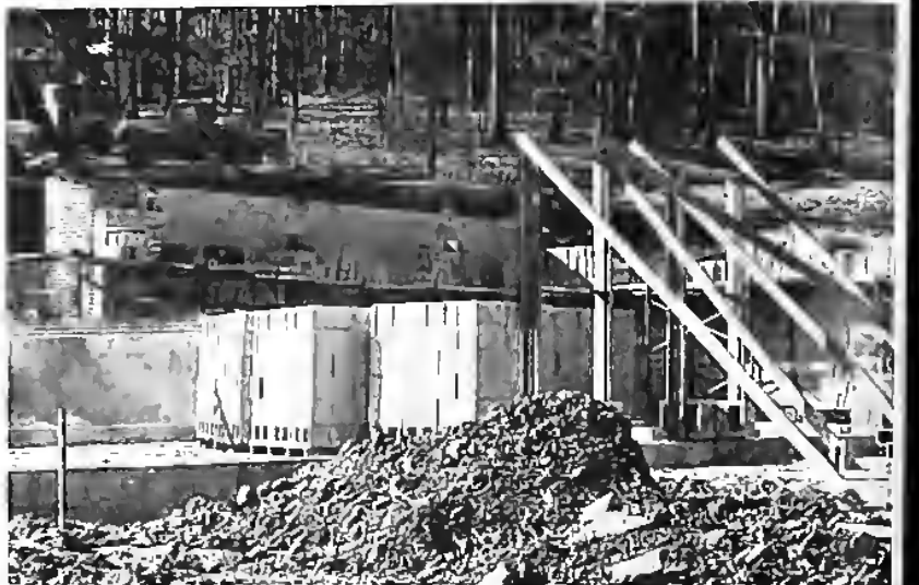
The old, abandoned Collegedale Academy building has been razed to make way for the new home economics center, now under construction.
