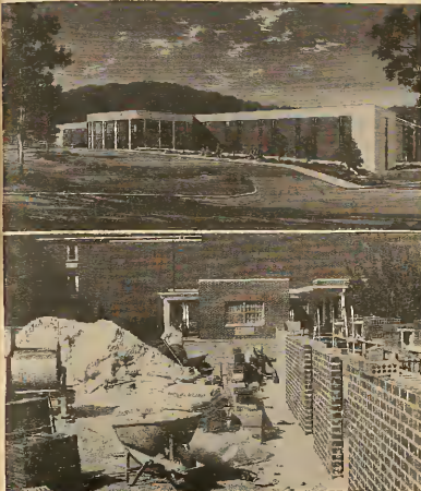
Construction is in progress (bottom photo) on the proposed new addition to the women's residence hall (top photo). [courtesy of Public Relations office]
