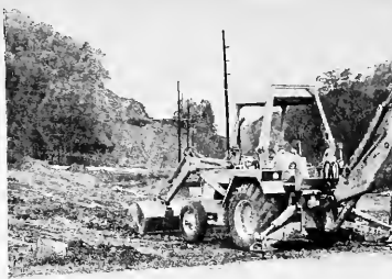
Construction is progressing on Hickman Hill Road. It appears that the road may be closed permanently for public use in the near future. (Photo by Sharon Webster).
