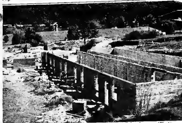
Construction on the new dorm addition to Thatcher Hall has begun. (Photo by Sharon Webster)
