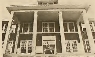
Lynn Wood Hall as it appeared last week. The building is nearing the end of a $100,000 renovation project funded by the Committee of 100.
