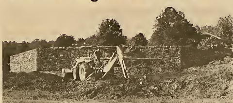
Neil Sorenson digs a trench in front of the new Southern College sign along Apison Pike
