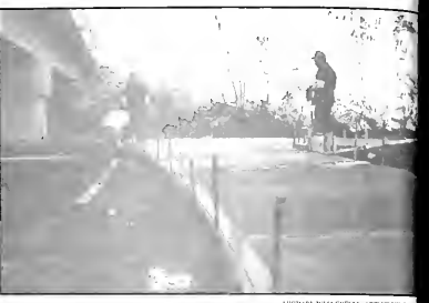
Construction is now underway on Collegedale's Greenway project (see the print page one for scaled plans of a walkway).
