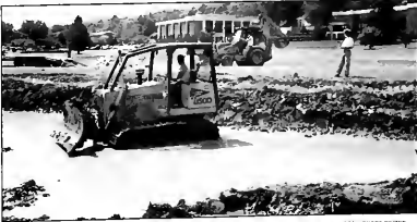
Contractors work on dredging the duck pond last week. Landscape Services said dredging must be done occasionally because of sediment build-up.
