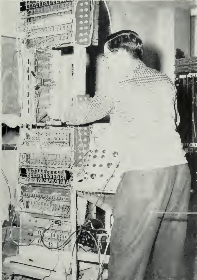
Student learns the intricacies of wiring some of modern equipment that the College has procured for extensive work.
