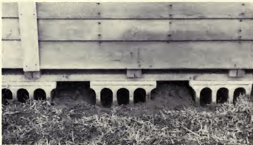
Blocks were placed at right angles with the floor joists under large bins, and a 2-by-6-inch sill was laid across the blocks to keep both the blocks and the joists from tipping. (Fig. 20)
