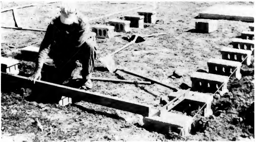
Concrete blocks with the cores horizontal were leveled to make temporary foundations for small bins. (Fig. 19)
