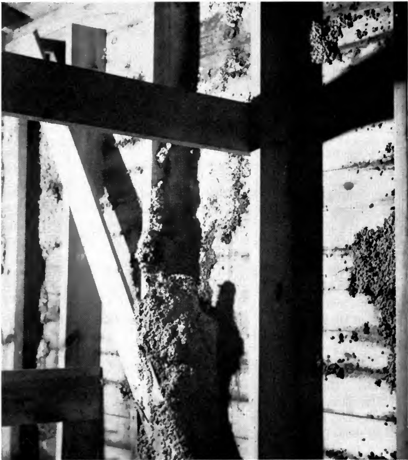
Leaks resulted in damaged soybeans on the inside of bin walls. Reinforced paper lining was not enough to prevent such damage. (Fig. 25)
