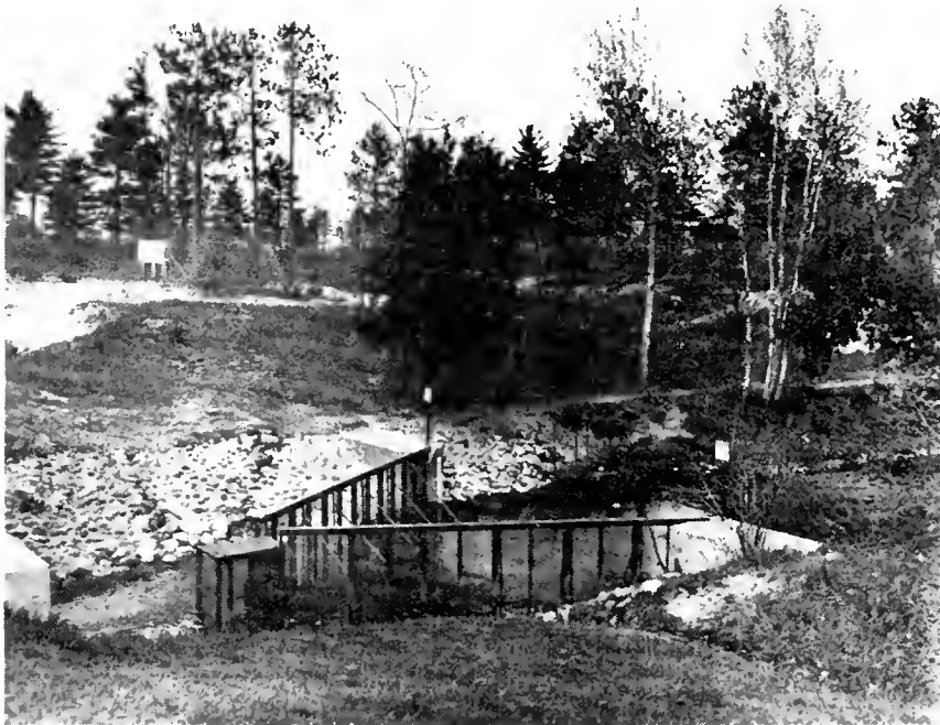
Figure 5.--Portable-type weir and trap in Carp Creek, Presque Isle County, Mich., after installation of permanent sills, trap base, and abutments of concrete.
