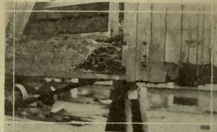
Decay in untreated boxcar sill
