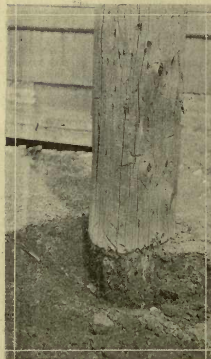
Untreated pole destroyed by decay
