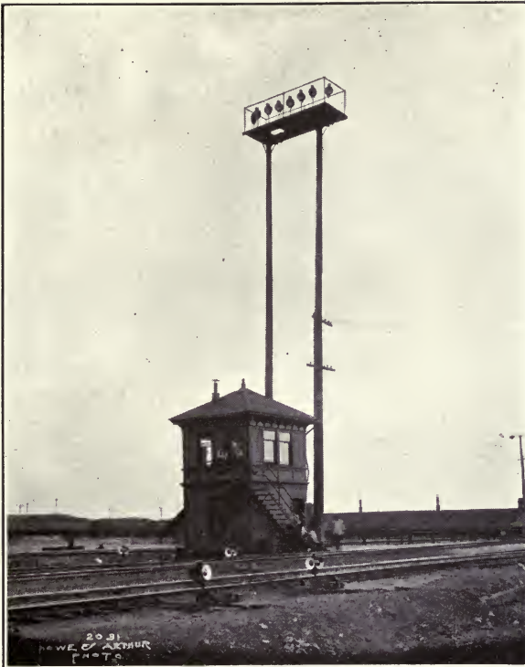
Pennsylvania Freight Yards, Chicago—Two-pole tower mounting eight 1000-watt Floodlight Units. Two such towers are employed 3000 feet apart, with beams opposed.
