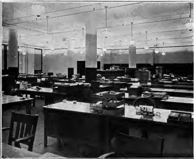
Common Sense Office Lighting of a Modern Type. 150-watt clear MAZDA C lamps are used on 10 ft. centers, 4 outlets per bay. The resultant illumination is slightly over 9 foot-candles
