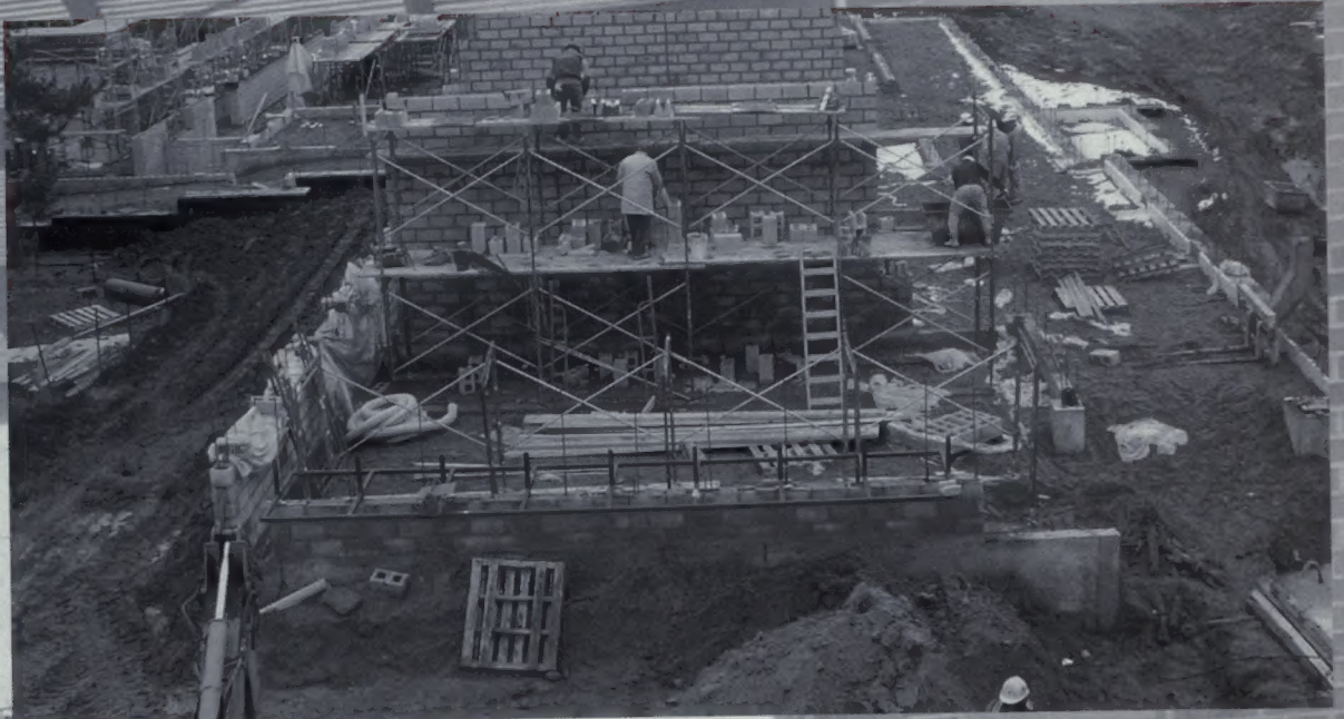
At this point the foundation has been laid for the new middle school.
