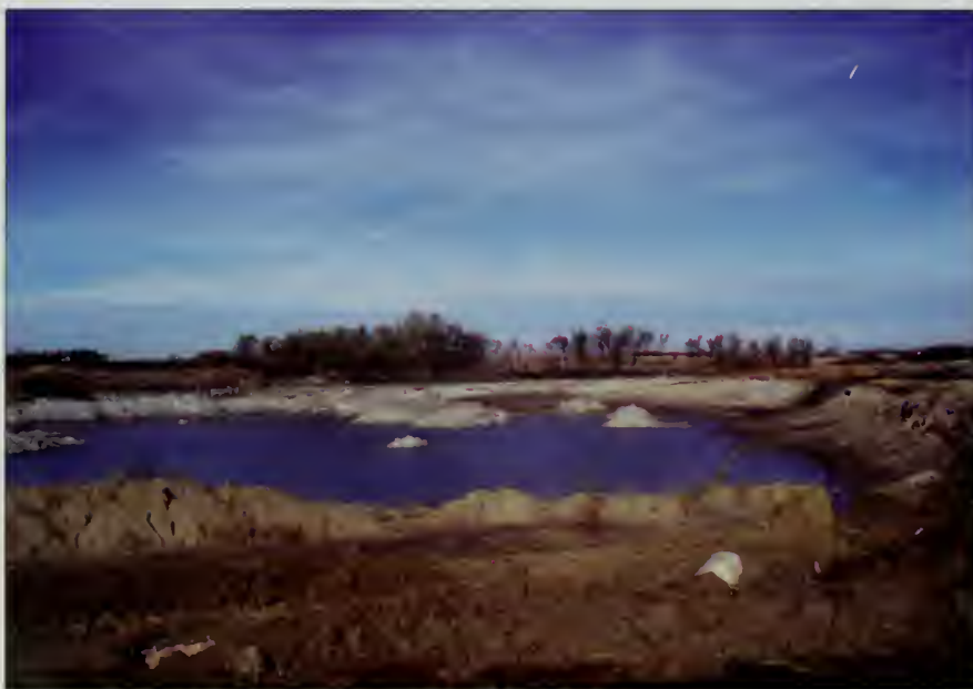
Figure 13. Lands in transition from one land use category to another pose unique challenges for image analysts. Field inspection of this site indicated the area was under construction as part of a highway project.
