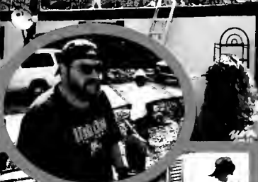
Chelsea O'Connell, Andrew Higgin, Amy Deering, and Amy Foulkes worked to put tar on Jamie and Megan Price's roof.
