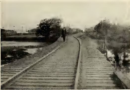
THE RAILROAD TRACK THAT SLIPPED.
