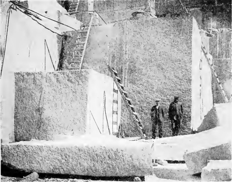
FIG. 25.—Granite quarry at Barre, Vt., in which various methods of drilling are illustrated. (Courtesy of E. L. Smith & Co.)
