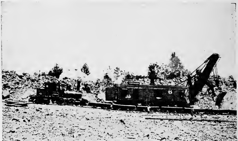
FIG. 71.—A large railroad-type shovel loading limestone into cars hauled by steam locomotive.
