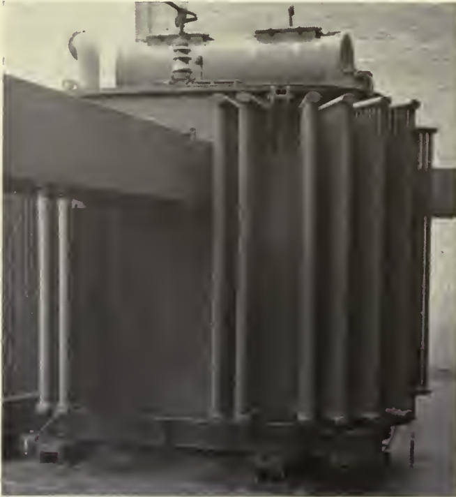
5,000-KVA Power Transformer installed at Harrisburg Steel Corporation Plant.
