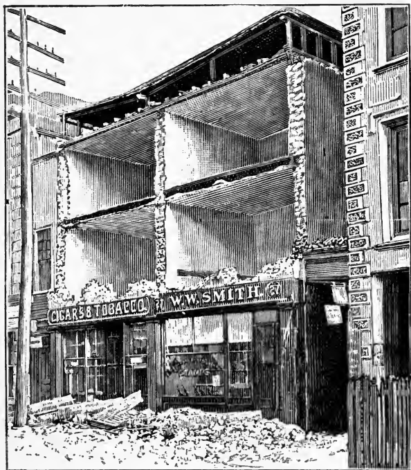
FIG. 110.—STREET HOUSES IN CHARLESTON DAMAGED IN THE SOUTH CAROLINA EARTHQUAKE OF 1886.
