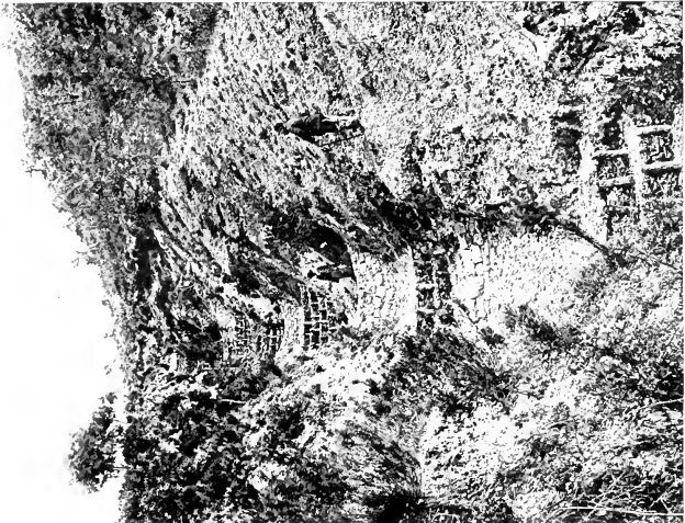
FIG. 10 (c). — Log and dry stone dams to prevent further erosion at Var-Moyen (Alpes-Maritimes). (French official photograph.)
