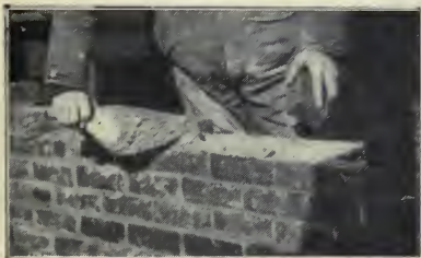
Fig. 26. — Buttering the end of the laid brick on the exterior face tier.
