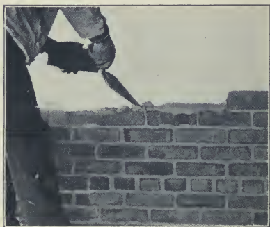
Fig. 33. — Handling mortar for two brick at one time on interior face tier.
