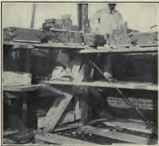
Fig. 1.— Non-stooping scaffold designed so that uprights are out of the bricklayer's way whenever reaching for brick and mortar at the same time.
