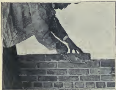
Fig. 32. — Cutting off mortar after brick is laid on interior face tier (here working left to right).
