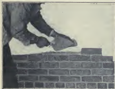
Fig. 42.—Working right to left.—Buttering right-hand end of brick in hand to be laid on interior face tier.
