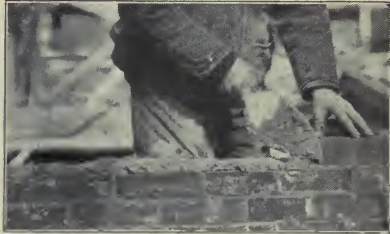
Fig. 35.—Working left to right.—Buttering end of laid brick on exterior face tier.
