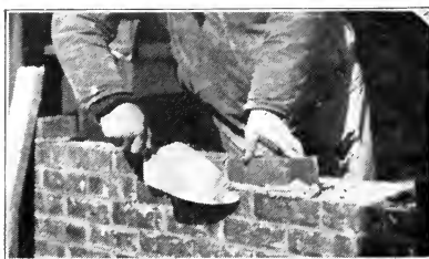
Fig. 27. — Cutting off the mortar after the brick is laid on the exterior face tier.
