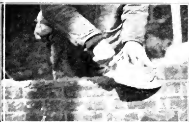
Fig. 36.—Working left to right.—Cutting off mortar after brick is laid on exterior face tier.
