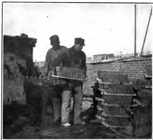
Fig. 3.—Arrangement of gravity conveyor for unloading brick so that laborer does not have to stoop.
