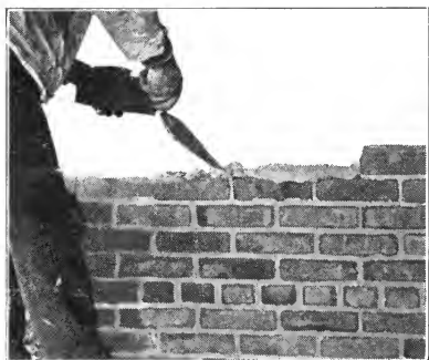
Fig. 33. — Handling mortar for two brick at one time on interior face tier.
