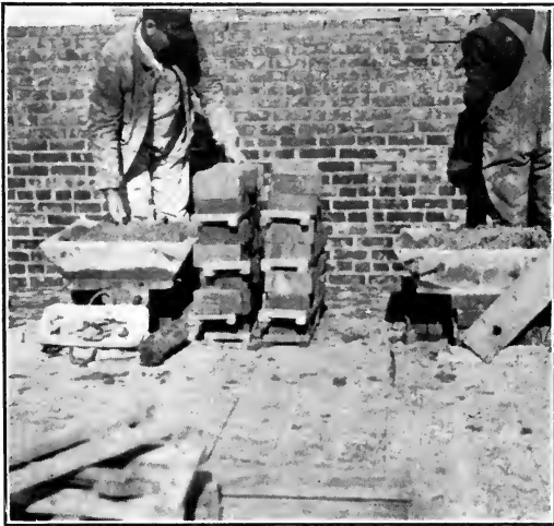
Fig. 12. — Standard practice for providing bricklayers with material for pick-and-dip method of bricklaying when the wall is shoulder high.
