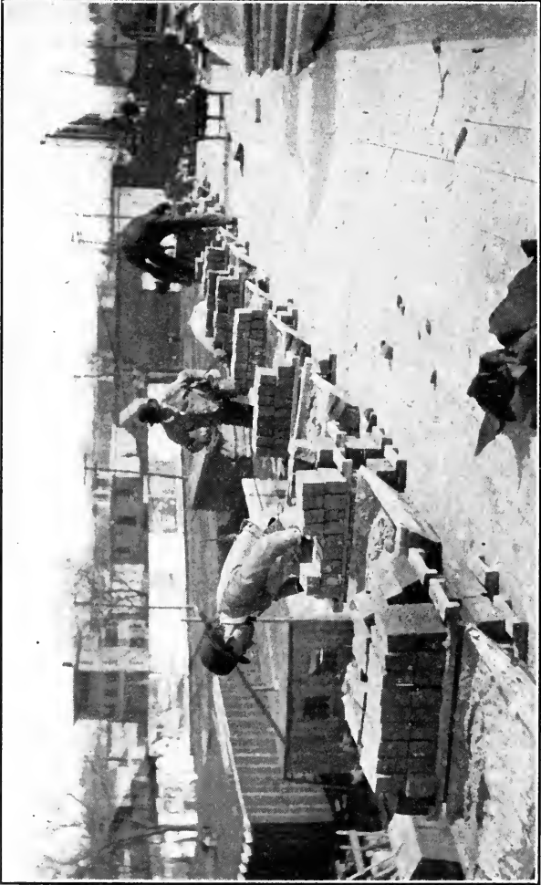
Fig. 10.—Standard practice of providing bricklayers with materials—mortar boxes on the floor and low piles of packs when the wall is below the level of the top of the floor.
