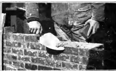
Fig. 25. — Cutting off mortar before the brick is laid on exterior face tier.
