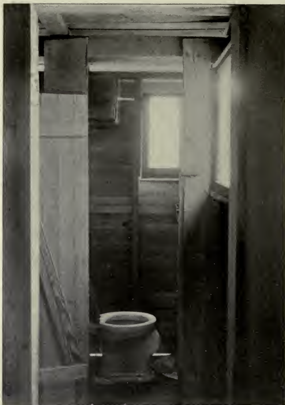
FLIMSY CONSTRUCTION OF COMPARTMENTS, AND POOR INSTALLATION OF PLUMBING. TOILET SEAT BROKEN OFF (SECOND TOILET AT LEFT). DWARF DOORS, INADEQUATE PRIVACY, AS TWO TOILETS ARE USED BY BOTH SEXES (SEE NEXT PICTURE FOR OUTSIDE CONSTRUCTION)
