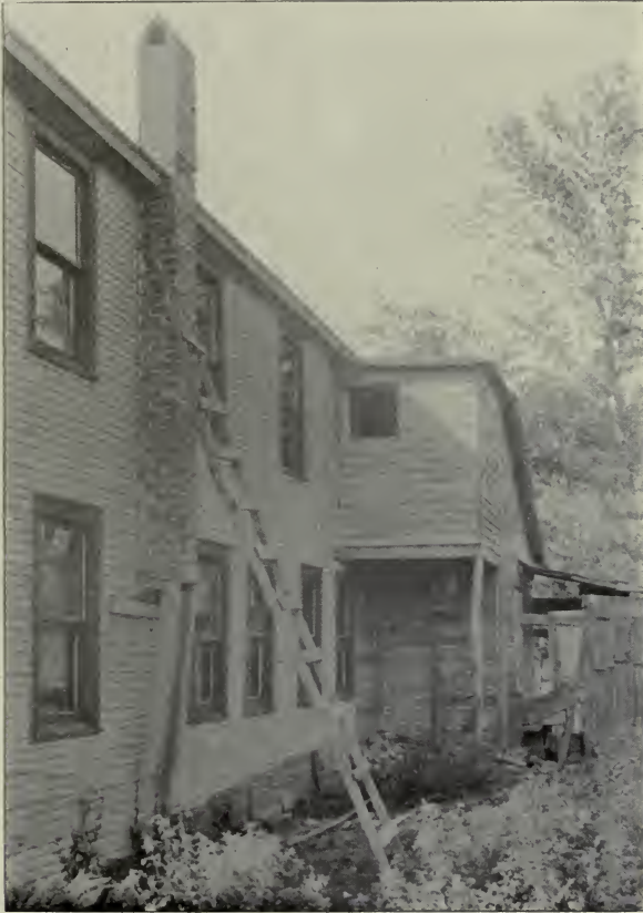
WATER CLOSET IN EXTENSION (TWO COMPARTMENTS) SUPPORTED BY POLE. NOTE ALSO CHIMNEY SUPPORTED ON BRACKET
