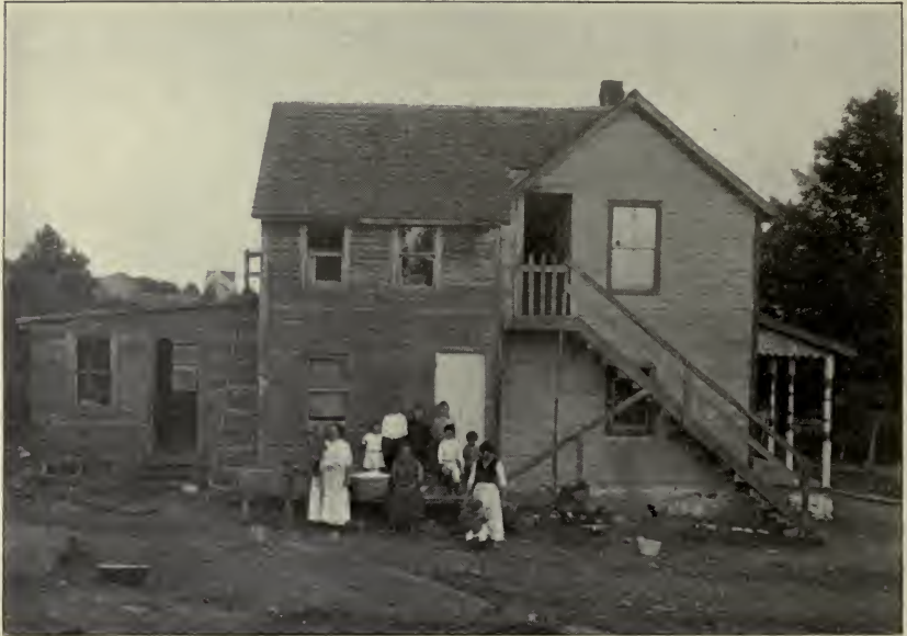
FLIMSY ADDITIONS, THIN PARTITIONS BETWEEN UPSTAIRS BEDROOMS. ONE WINDOWLESS ROOM ON FIRST FLOOR. EXTENSION IN REAR COMBINED KITCHEN AND DINING ROOM FOR 10 FAMILIES. OUTSIDE STAIRS UNSAFE
