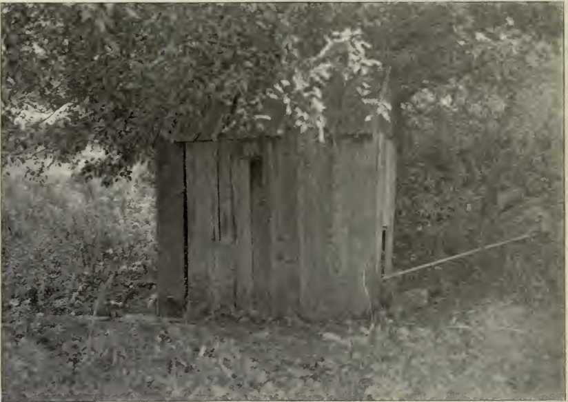
SHELTER OVER SPRING AT FOOT OF HILL. BOARDS OF SHELTER ROTTED AT BOTTOM. GROUND AROUND SPRING, DEEP MUCK. SPRING ONLY WATER SUPPLY FOR 10 FAMILIES IN HOUSE. RECEIVES SURFACE DRAINAGE FROM YARD. TWO PRIVIES AND KITCHEN SINK
