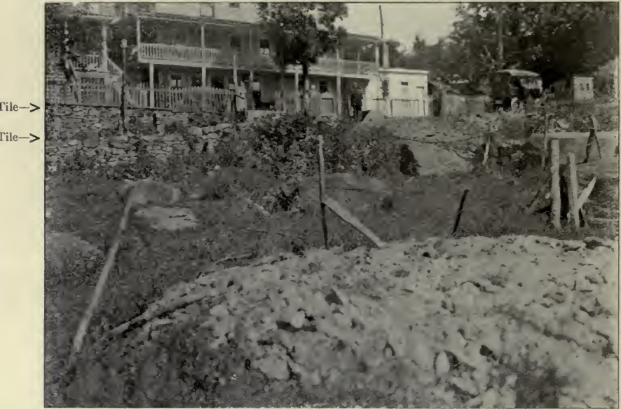
SEWAGE DISPOSAL FOR LARGE BOARDING HOUSE. TILE COMES THROUGH TWO WALLS WITH ROAD BETWEEN AND IS CARRIED ON TOP OF GROUND TO SHALLOW HOLE IN A SWAMPY SPOT. SEWAGE LEAKS THROUGH AND SPREADS OVER FIELD ABOUT 50 FEET FROM HOUSE
