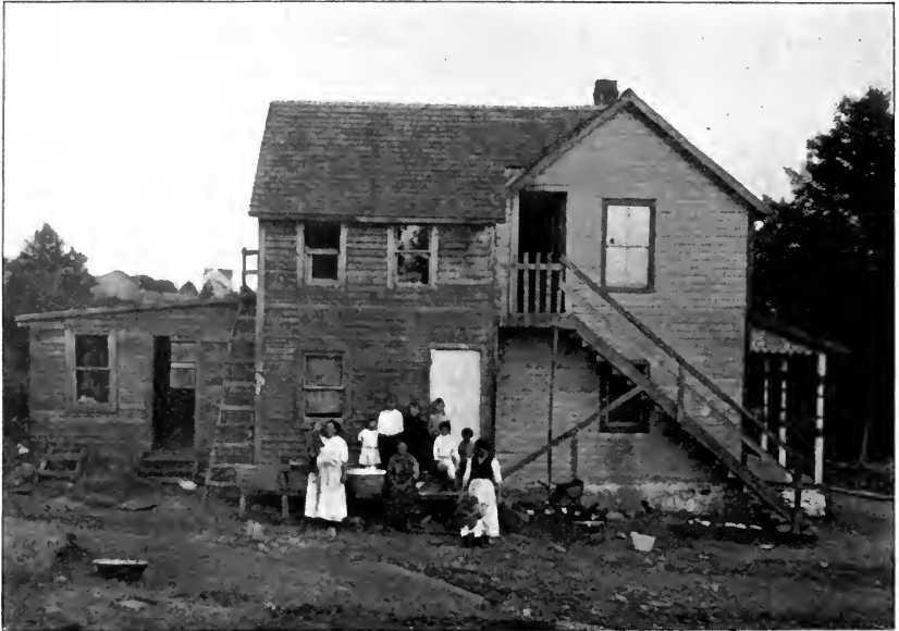
FLIMSY ADDITIONS, THIN PARTITIONS BETWEEN UPSTAIRS BEDROOMS. ONE WINDOWLESS ROOM ON FIRST FLOOR. EXTENSION IN REAR COMBINED KITCHEN AND DINING ROOM FOR 10 FAMILIES. OUTSIDE STAIRS UNSAFE
