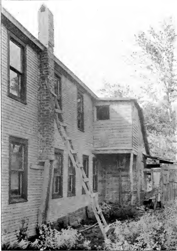
WATER CLOSET IN EXTENSION (TWO COMPARTMENTS) SUPPORTED BY POLE. NOTE ALSO CHIMNEY SUPPORTED ON BRACKET
