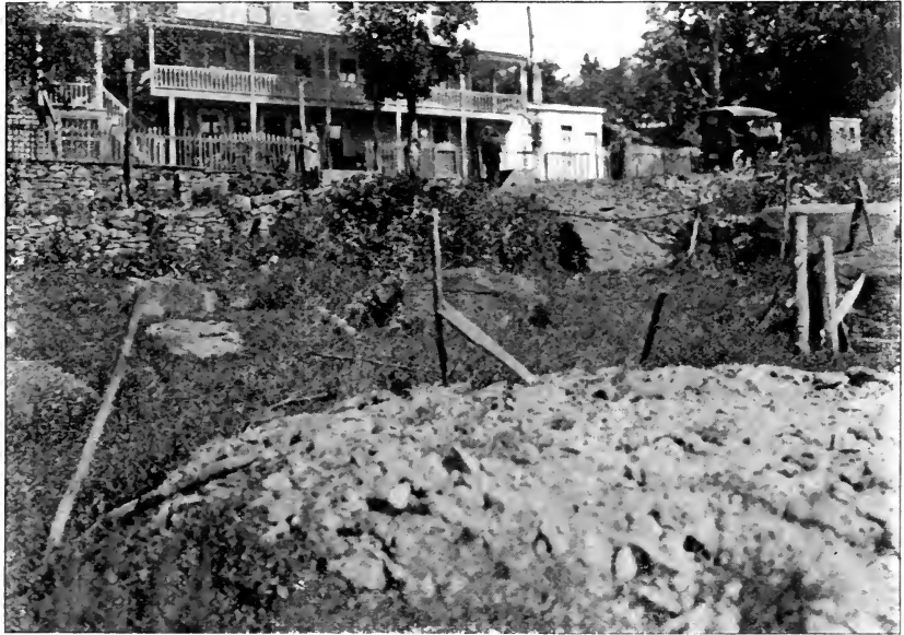
SEWAGE DISPOSAL FOR LARGE BOARDING HOUSE. TILE COMES THROUGH TWO WALLS WITH ROAD BETWEEN AND IS CARRIED ON TOP OF GROUND TO SHALLOW HOLE IN A SWAMPY SPOT. SEWAGE LEAKS THROUGH AND SPREADS OVER FIELD ABOUT 50 FEET FROM HOUSE
