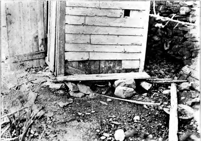
PRIVY SET ON TOP OF GROUND. NO REMOVAL BOX OR PAILS. FECAL MATTER OVERFLOWING ON GROUND OUTSIDE. SATURATION FOR FOUR FEET. USED BY AT LEAST 24 PERSONS ALL SEASON
