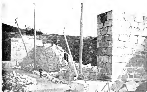
ISLAND POND ELECTRIC Co.'s DAM AT WEST CHARLESTON IN COURSE OF CONSTRUCTION.
