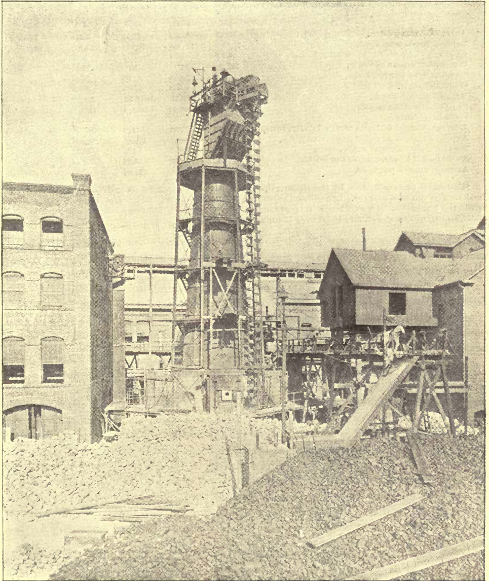
This building at the left is for the Steffens process of refining.
