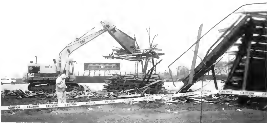
A construction crew cleared former stands on Amos Alonzo Stagg Field to prepare the site for the sports fitness project that will include the new Lopardo stadium, the Jacobs Fitness Center and a 51,000-square-foot field house.
