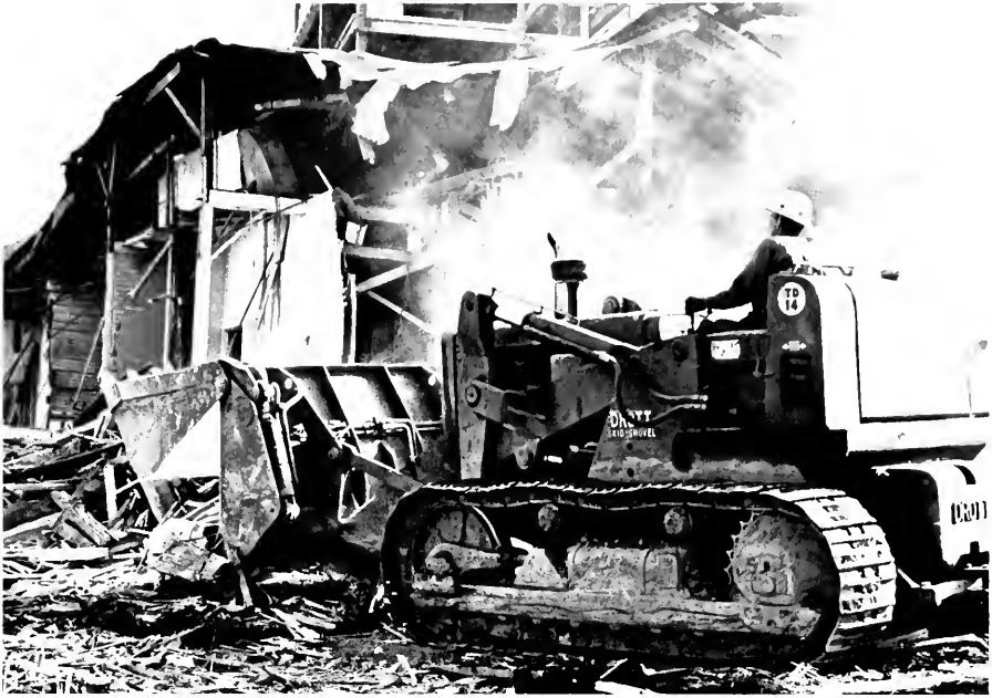
A bulldozer makes way for a new dormitory by removing the vacated "old" McCabe Building.
