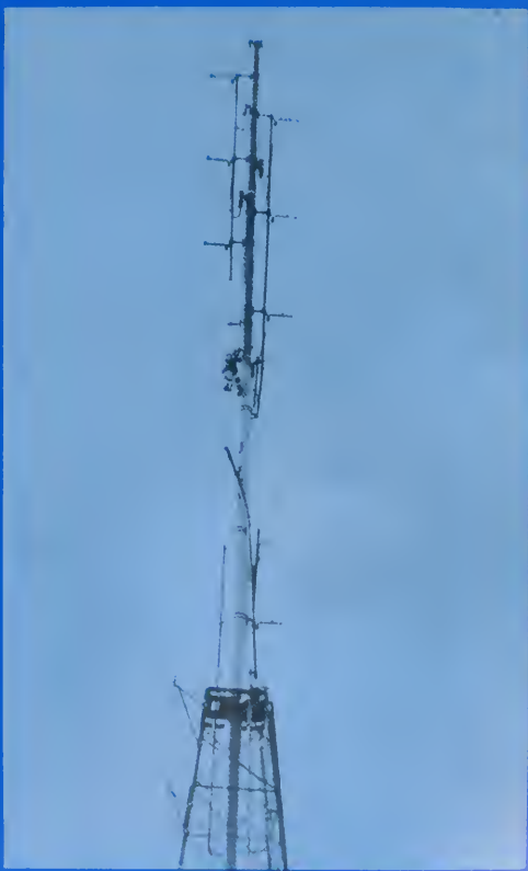
The WAMU tower was surprisingly not sheared completely off, but was heavily damaged. Many students feel that it was the tower that kept the plane from striking the Letts-Anderson complex.
