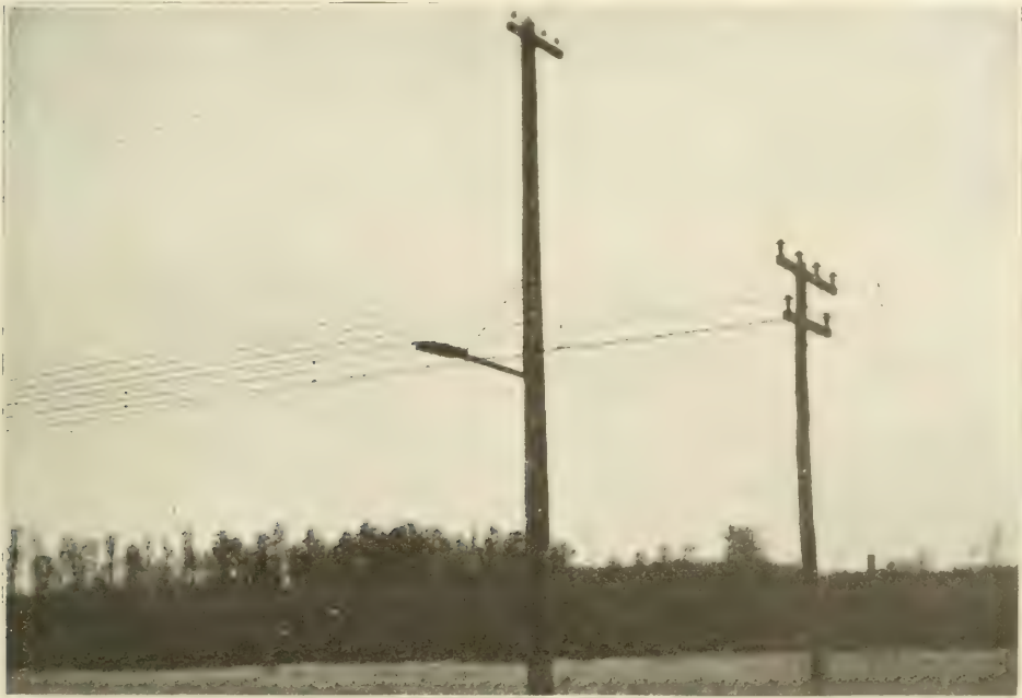
OVERHEAD CONSTRUCTION SHOWING CATENARY SUSPENSION.
