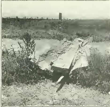
A SMALL TWO BY TWO CONCRETE CULVERT WOULD OBLIATE THIS VERY COMMON DISGRACE.
