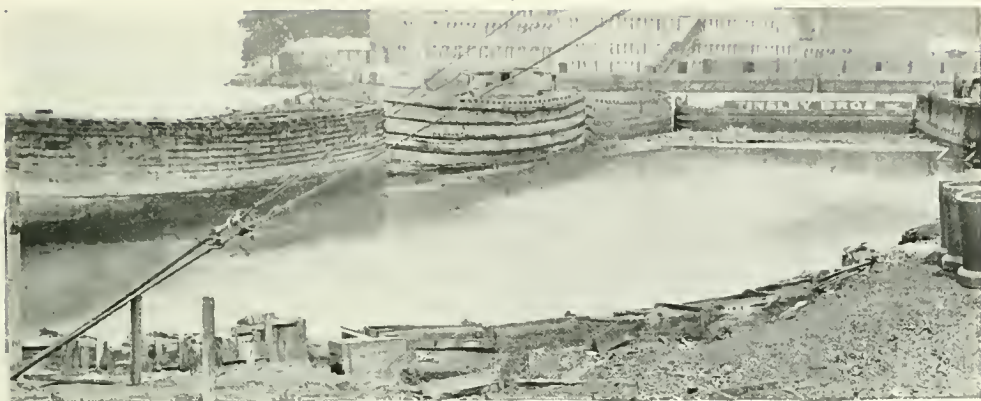
BARGES AS BASIS FOR FACTORY SITE. A string of worn-out craft that an enterprising contractor is using.
