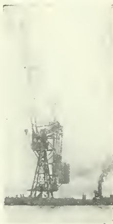
THE CRANE ON THE WATER. This monster is capable of lifting two hundred tons.
