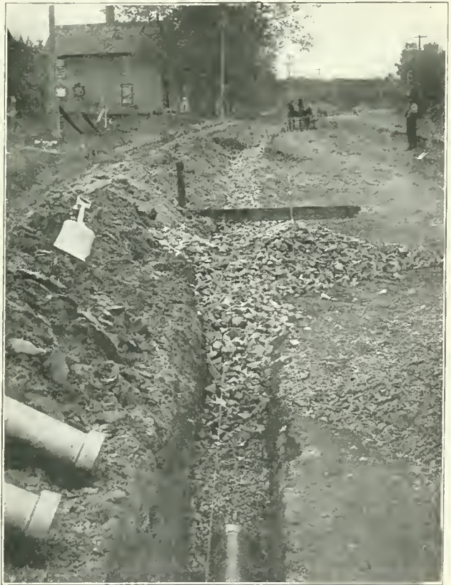
MILES OF THIS TYPE OF DRAIN OUGHT TO BE BUILT ALONG OUR HIGHWAYS. Laying side drains at Westfield, Mass.
