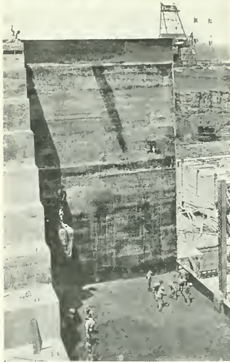
AT WORK ON THE GATUN DAM, PANAMA. Placing the concrete that forms huge monolithic walls for the dam.
