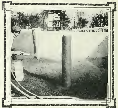
BUILDING UP A SECTION OF CEMENT PIPE ON A WIRE MESH SKELETON OR REINFORCEMENT. A cement-gun-made fence is shown in the background.
