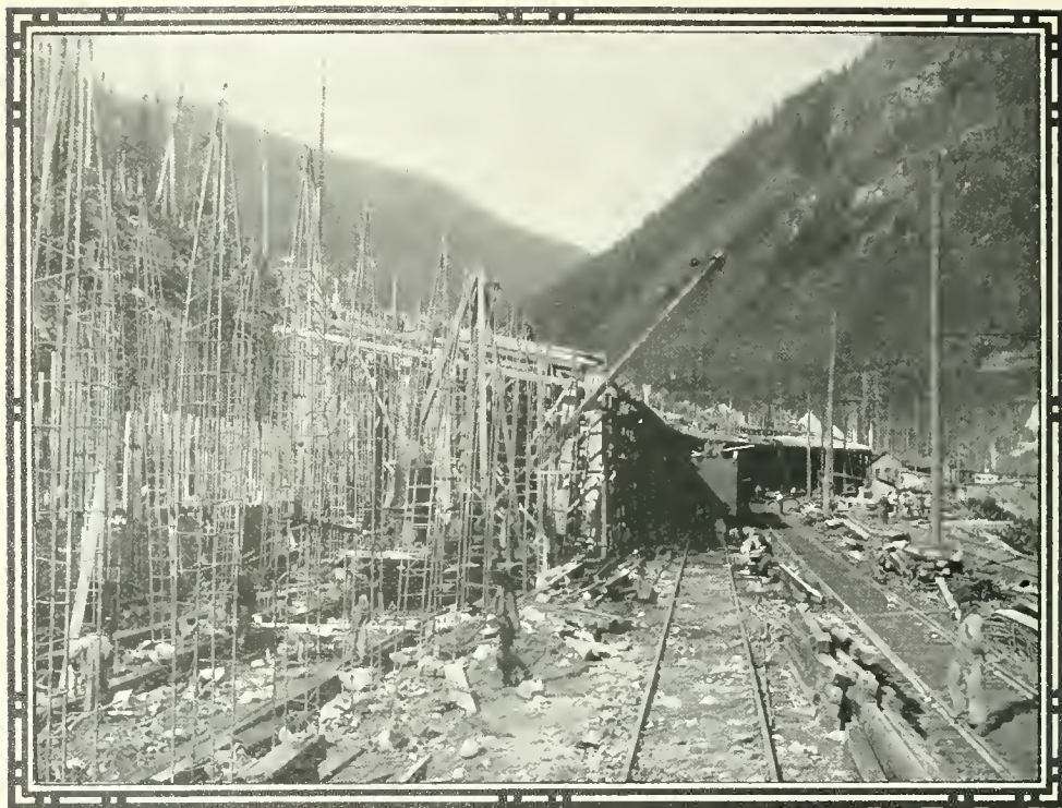
WHERE ONE HUNDRED PERSONS LOST THEIR LIVES. Building concrete sheds to protect from snow slides at Wellington, Washington.
