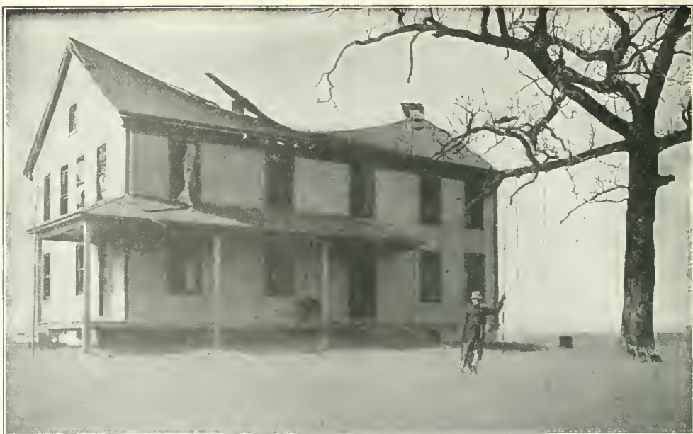
AS THOUGH IT HAD BEEN STRUCK BY THE LOOSE END OF A TORNADO. A dwelling three-fourths of a mile distant from Pleasant Prairie.
