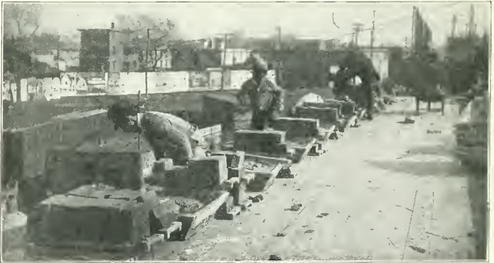
THE RIGHT WAY—IMPROVED METHOD OF HAVING THE BRICKS ON PACKETS AND THE BOXES PROPERLY SPACED FOR THE GREATEST SPEED WHEN THE WALL IS AT THIS LEVEL.
