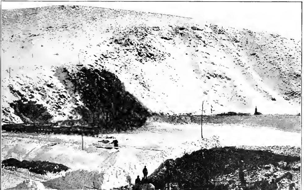
THE EXCAVATION WORK IN THE HILLSIDE, WHERE, LATER, ROCK WAS SET INTO ROCK. View of the gorge at the dam site.
