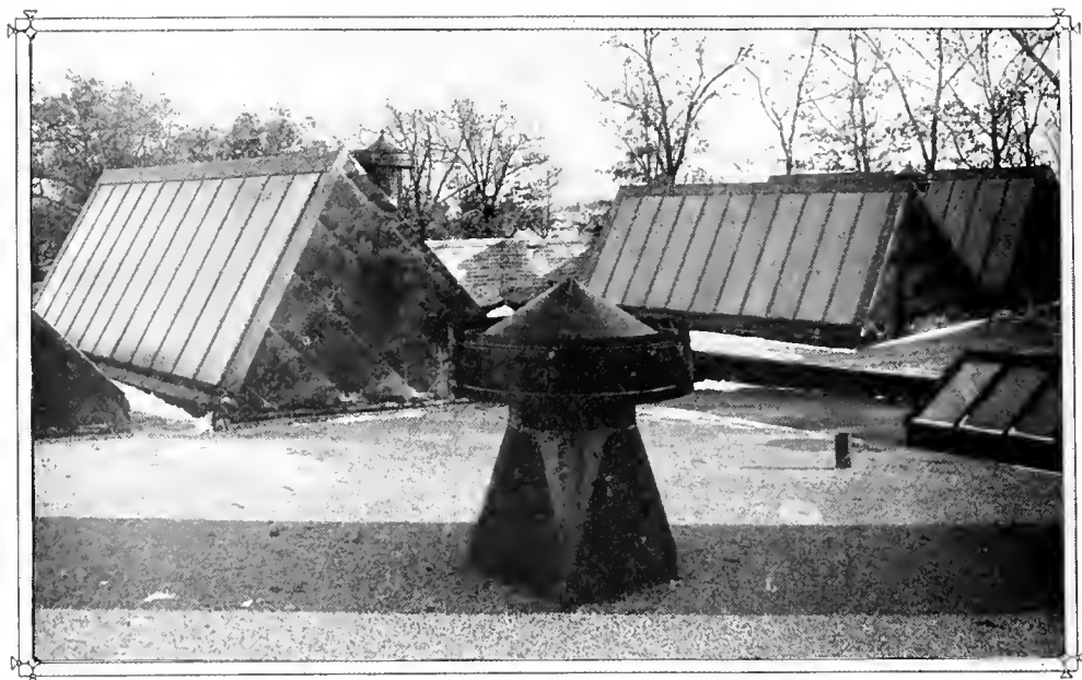
THE SAW-TOOTHED SKYLIGHTS WHICH ARE PARALLEL RIDGES RUNNING EAST AND WEST. The south slope is covered with tin, the north is of reinforced ribbed glass. Thus a steady north light is assured.
