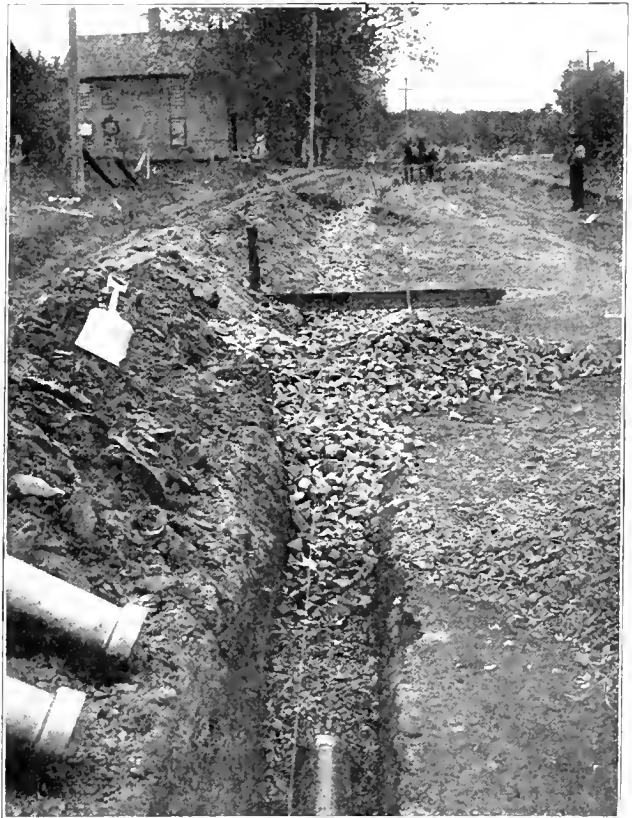
MILES OF THIS TYPE OF DRAIN OUGHL TO BE BUILT ALONG OUR HIGHWAYS. Laying side drains at Westfield, Mass.
