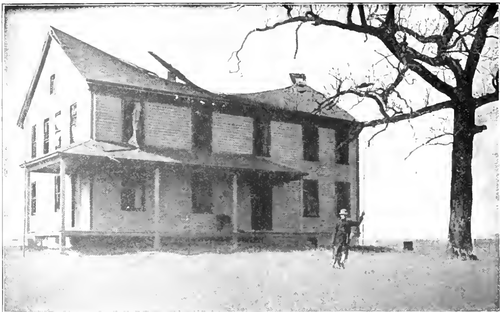
AS THOUGH IT HAD BEEN STRUCK BY THE LOOSE END OF A TORNADO. A dwelling three-fourths of a mile distant from Pleasant Prairie.
