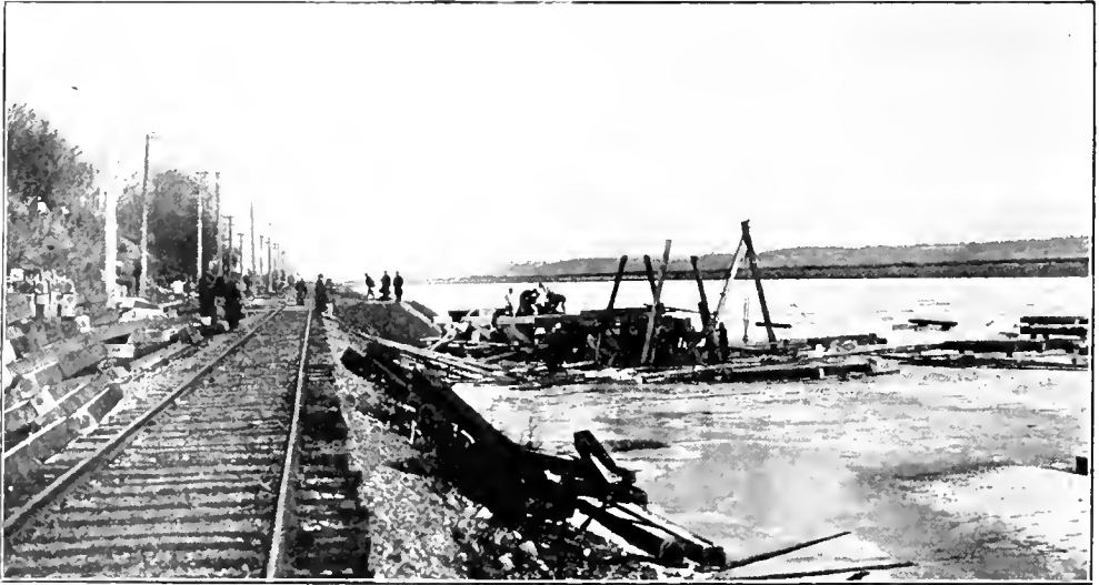
BUILDING A BRIDGE TO THE ILLINOIS SHORE. The beginning of work on the Iowa side.
