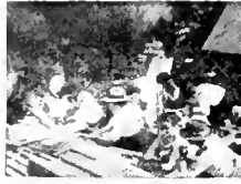
PUTTING ON SHINGLES. Here the ladies of the church found more employment.
