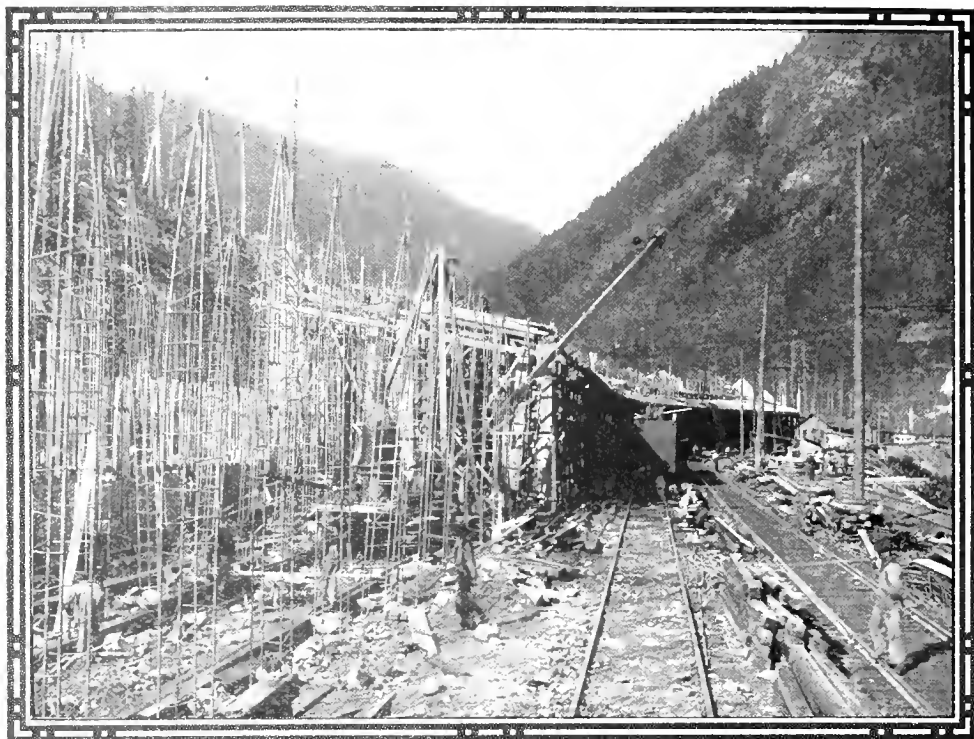
WHERE ONE HUNDRED PERSONS LOST THEIR LIVES. Building concrete sheds to protect from snow slides at Wellington, Washington.
