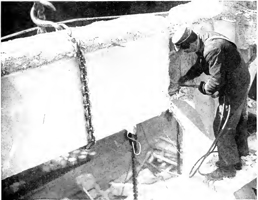
CUTTING A GIRDER IN TWO WITH A BLOW PIPE. The workman has a most limited space for footing.
