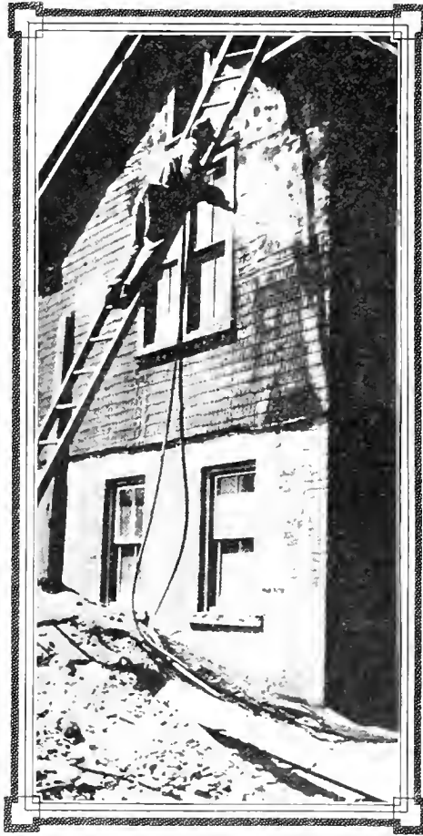
APPLYING CEMENT STUCCO TO AN OLD BUILDING AFTER COVERING IT WITH WIRE MESH
