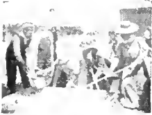
MIXING THE MORTAR. The women helped from the very beginning of the task.
