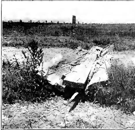
A SMALL TWO BY TWO CONCRETE CULVERT WOULD OBLIVATE THIS VERY COMMON DISGRACE.
