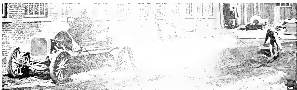
FOCAL TO SIX TEAMS OF HORSES. Automobile which proved its efficiency by excavating for a 5,000-gallon gasoline tank. There seems to be no end to the uses to which this pleasure machine may be put.
