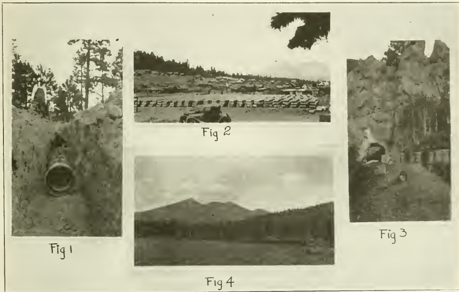
Figure 1—START OF CONCRETE PIPE LINE. Figure 2—VIEW OF STORAGE YARD FOR CONCRETE PIPE. Figure 3—TYPICAL TUNNEL THROUGH ROCK OBSTACLE. Figure 4—VIEW OF SAN FRANCISCO PEAKS OVER RESERVOIR.
