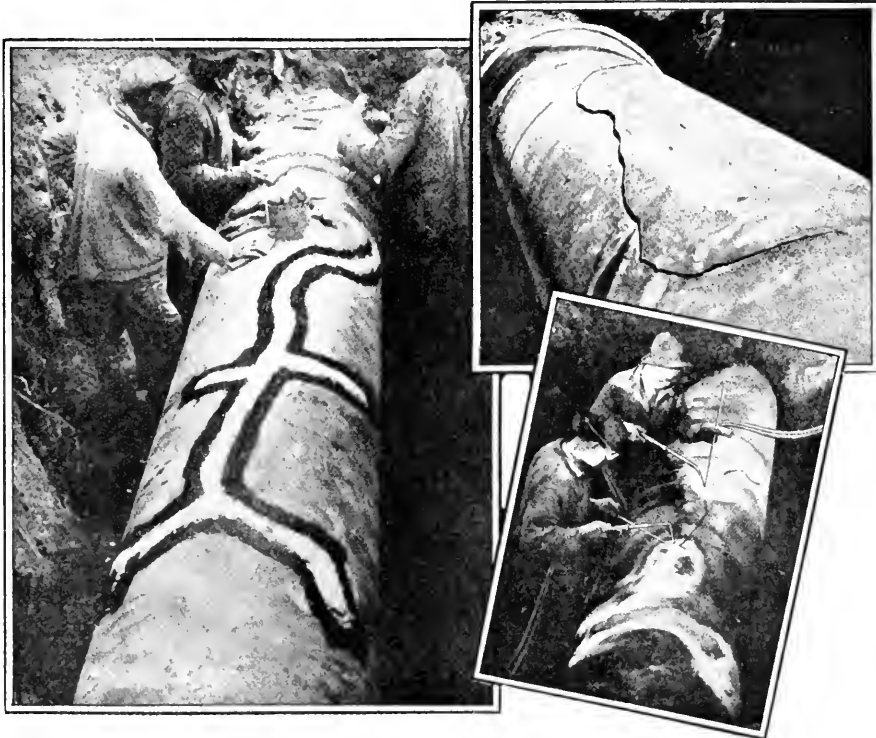
FIGURE 4.—ILLUSTRATIONS SHOW HOW TOBIN BRONZE WELDING RODS WERE USED TO SEAL A 13 FT. FRACTURE IN A WATER MAIN AT WASHINGTON, D. C. (Photo by Courtesy of American Brass Company.)
