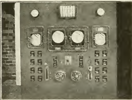
Bailey Meters on a Pulverized Coal Fired Boiler
