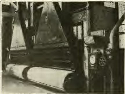
Bailey Meters at Western Electric Co., Kearney, N. J.
