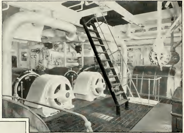
Typical engine room of a modern all-electric ship
