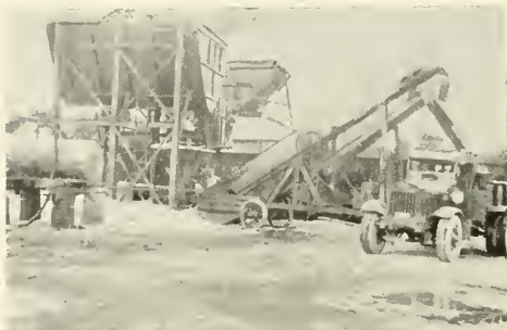
The central mixing and emulsifying plant where the materials for all the campus roads were proportioned and mixed
