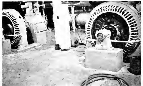
The two compressors in the engine room. Ammonia gas is compressed by these machines, then on expanding takes up heat from the brine pipes.
