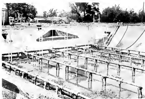
Settling basin, showing pipe system through which sludge is bled
