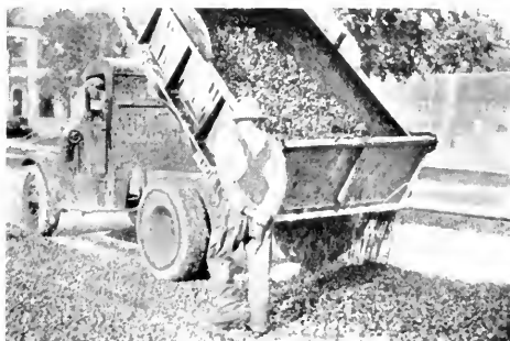
Pre-coted stone being dumped on the base on the new Sixth street surface
