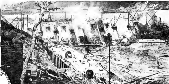
1902—Spier Falls Dam and Power Plant, Spier Falls, N. Y. Two #5 (2 yd.) Ransome Mixers used
