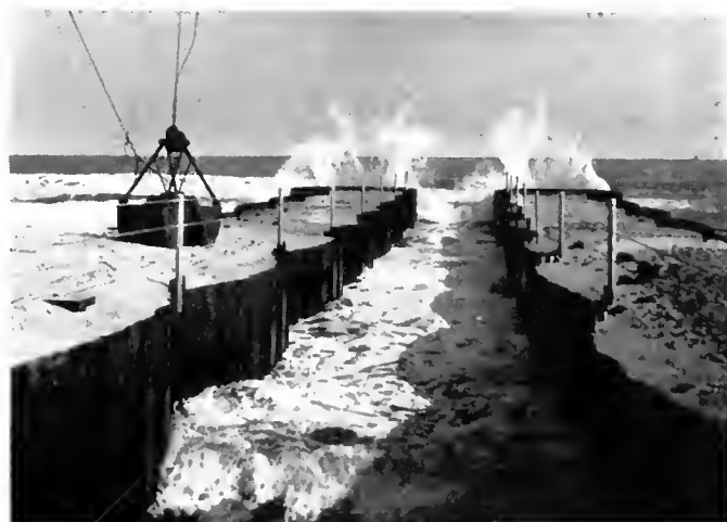
SEA WATER INTAKE
