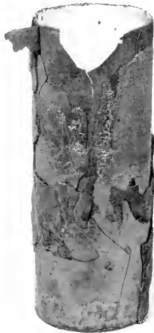
Typical heat-corrosion in an unprotected pipe
