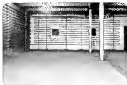
Storage Rooms Hold 300 Tons of Frozen Fish
