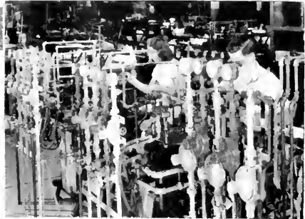
Over 40 miles of pipes deliver 13 needed services to working locations. These are hydrogen, oxygen, nitrogen, city gas, city water, deionized water, soft water (cold, hot, cooling) high pressure air, low pressure air, process steam and condensate return.
