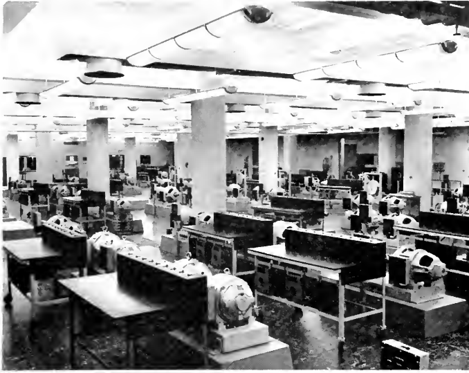
Room 50, the big basement motor-generator laboratory in the new E. E. building, is shown above. (Photo by Jack Chandler.)
