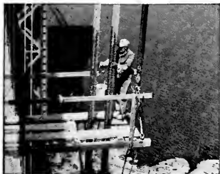
Rust would quickly weaken this structure. Because "Dulux" resists salt water and salt air, it has for years protected many famous bridges.
