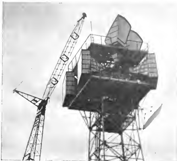
Microwave relay towers assure reliable land transmission of telephone, radio, television and data traffic—with complete flexibility.
