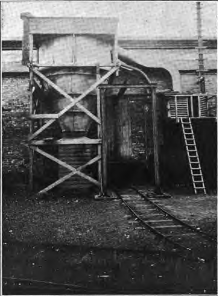
FIG. 40.—CYCLONE DUST COLLECTOR (NOBEL'S EXPLOSIVES Co.)
