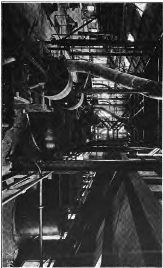
FIG. 12.—COTTON PURIFICATION BUILDING, TOP FLOOR (E. I. DU PONT DE NEMOURS Co.)
