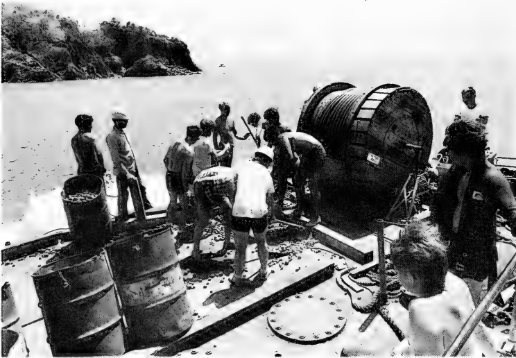
Figure 16. Drums of Ballast on Deck of Support Barge Being Shovelled into Tube Leading to Ballast Chambers in Base of TEKITE II Habitat.
