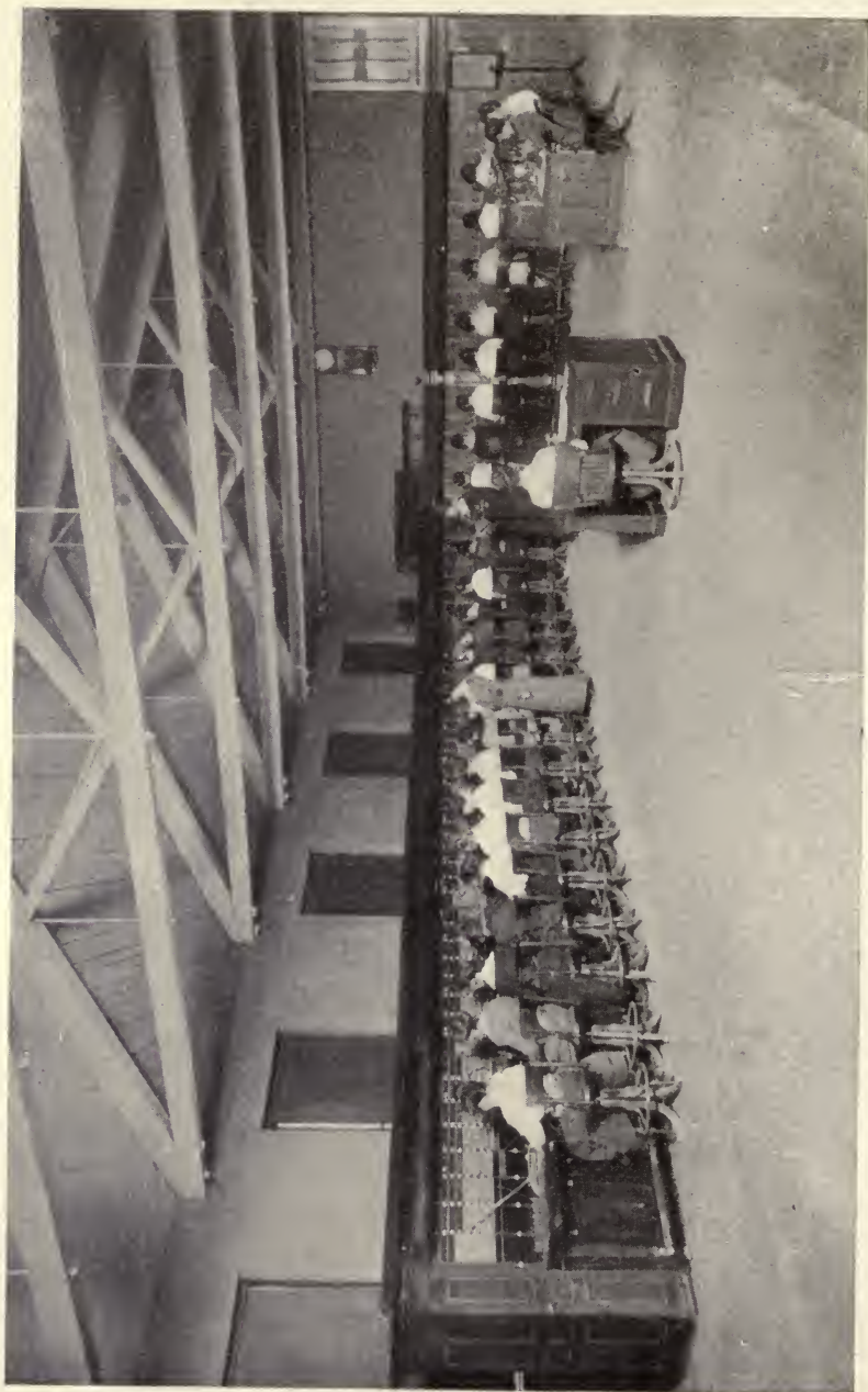
FIG. 55.—MULTIPLE SWITCHBOARD (Stromberg-Carlson)
