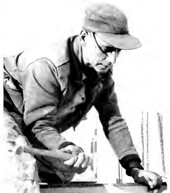
PHYSICAL PROGRESS of University is sounded out by carpenter at work on Administration Annex.
