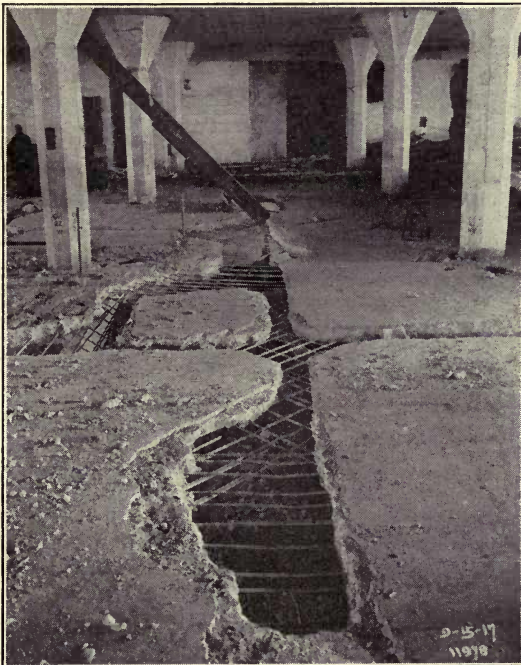
FIG. 21. VIEW OF SLAB AFTER REINFORCING BARS WERE EXPOSED
