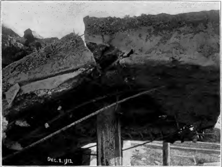
Fig. 11. Collapse of Norcross Slab
