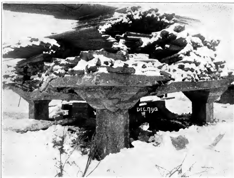
Fig. 18. Failure of Mushroom Slab.
