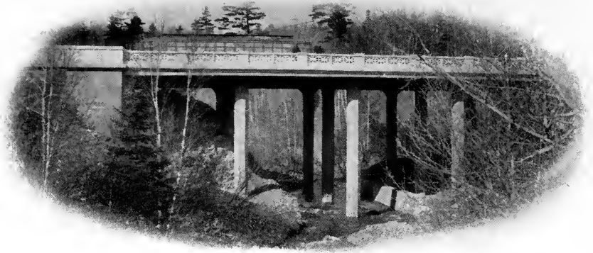
TISCHERS CREEK BRIDGE, DULUTH, MINN. Spans are 26 feet longitudinally This type is built with spans up to 50'0"
