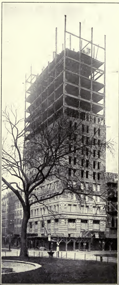
The steel framework of the Broadway Chambers Building, N. Y., was painted with Ebonite Varnish.
