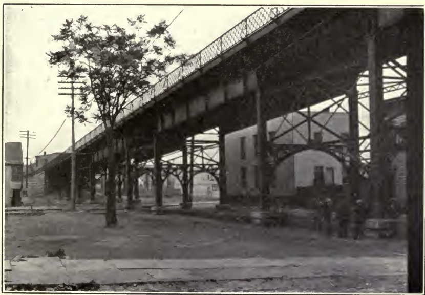
Highway Bridge at Albany, N. Y. Painted with Durable Metal Coating. Stowell and Cunningham, designers.
