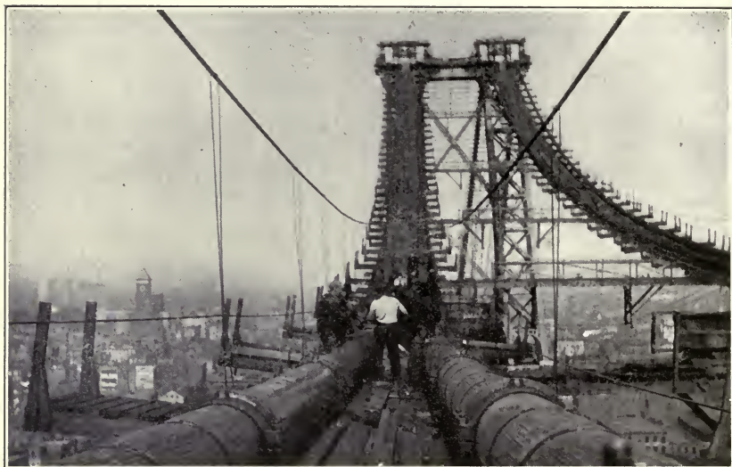
Applying Edw. Smith & Co.'s materials on the cables of the Williamsburg Bridge, N. Y. City.
