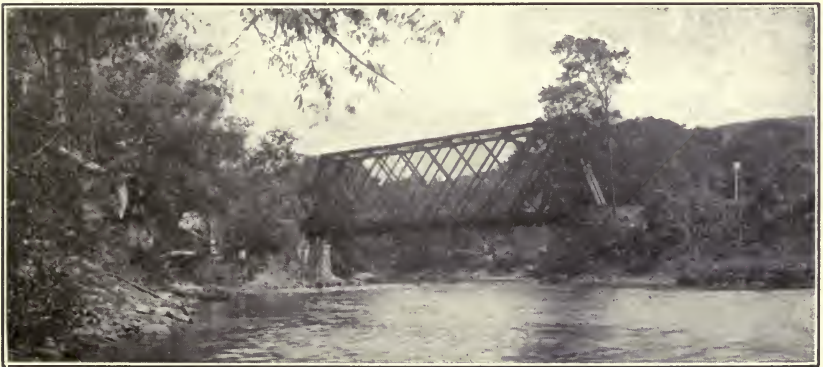
Eric R.R. bridge at Salisbury Mills, N. Y. Painted with Durable Metal Coating.
