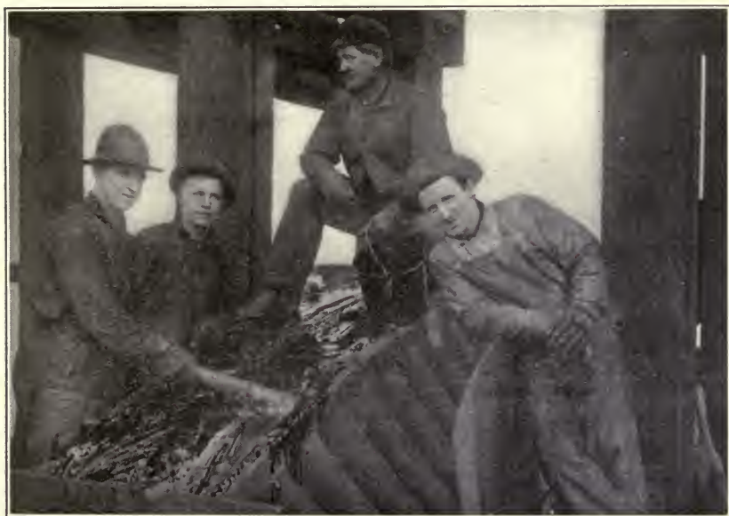
Applying Edward Smith & Co.'s materials on the saddles of the cables of the Williamsburg Bridge.
