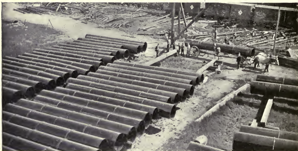
Thirty-eight-inch riveted steel pipe, Rochester, N. Y., 1893. Coated with Sabin Pipe Coating.
