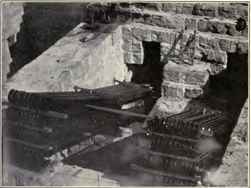
Eye-bar chains in the anchorages of the Williamsburg Bridge. Protected with Ebonite Varnish.
