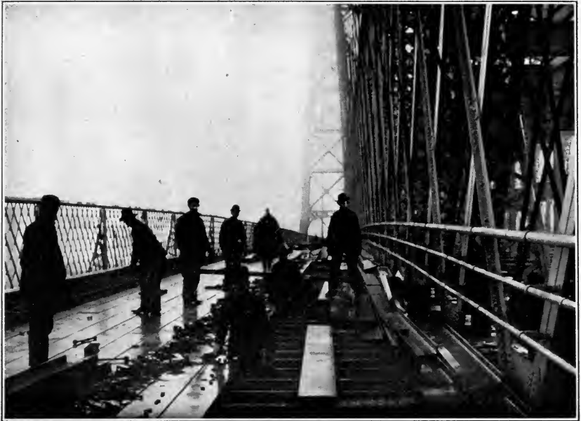
Laying the steel underfloor (coated with Sabin Pipe Coating) on the Williamsburg Bridge, N. Y. City.
