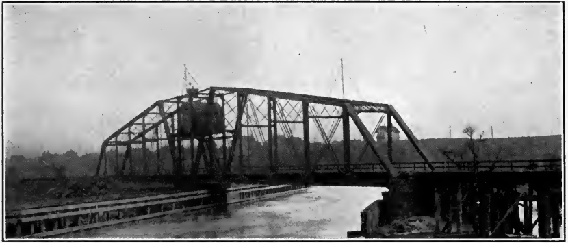
Drawbridge at Ashtabula Harbor, L. S. & M. S. R.R. E. A. Handy, Ch. Eng. Painted with Durable Metal Coating.
