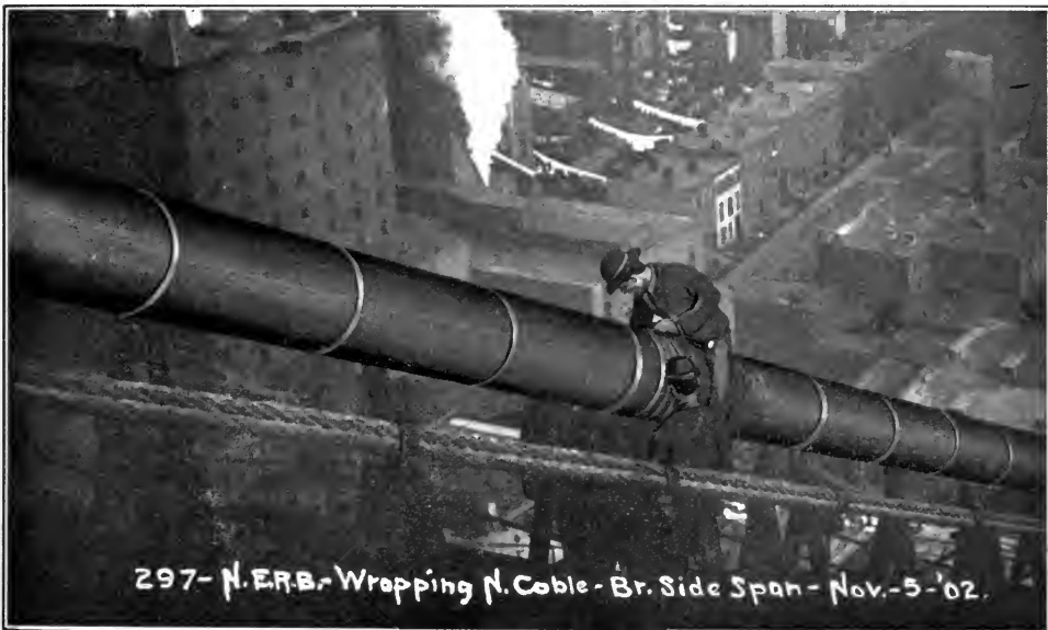
Applying Edw. Smith & Co.'s coating material on cables of Williamsburg Bridge, N. Y. City.
