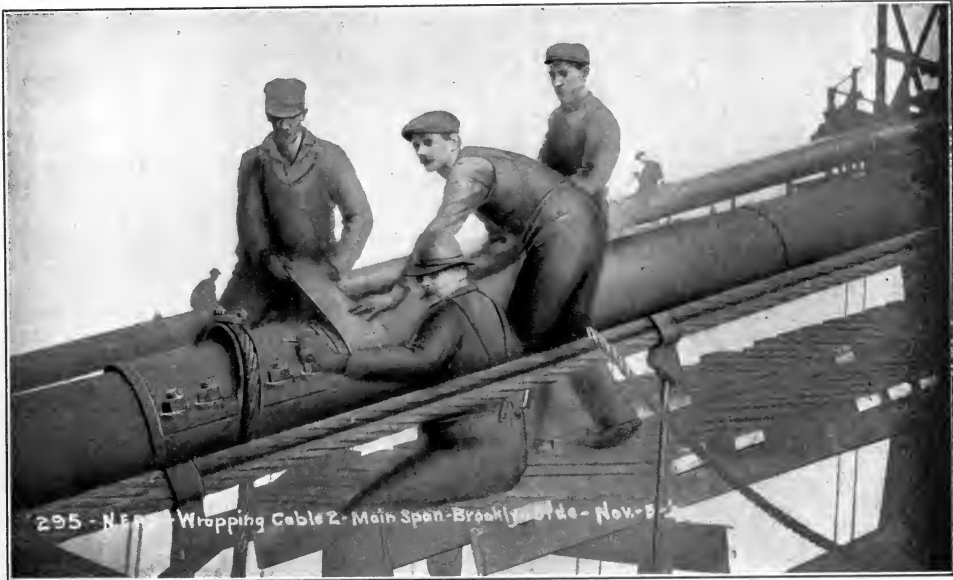
Applying Edw. Smith & Co.'s coating material on cables of Williamsburg Bridge, N. Y. City.
