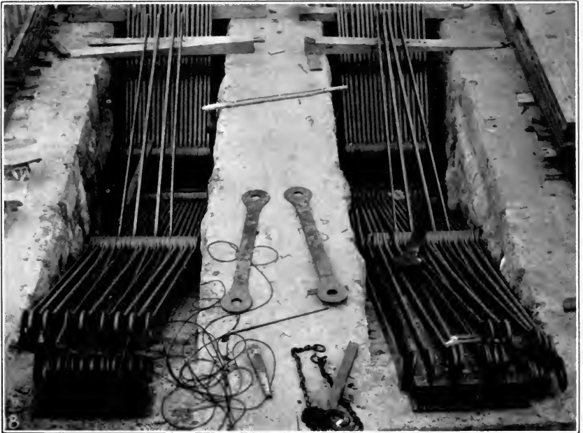
Eye-bar chains in the anchorages of the Williamsburg Bridge, N. Y. City. Protected with Ebonite Varnish.
