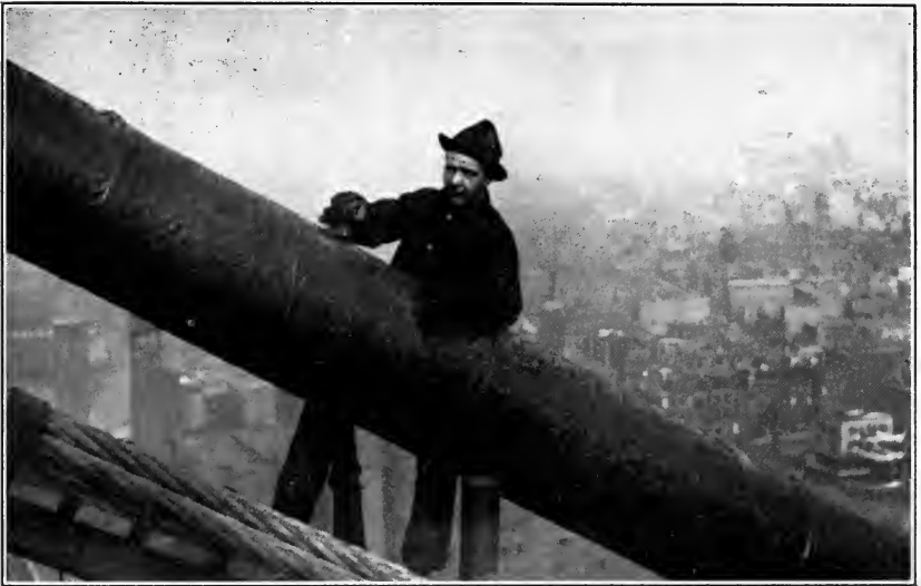
Using a hot iron in cementing the cable coating (design and material from Edw. Smith & Co.) on the Williamsburg Bridge, N. Y. City.
