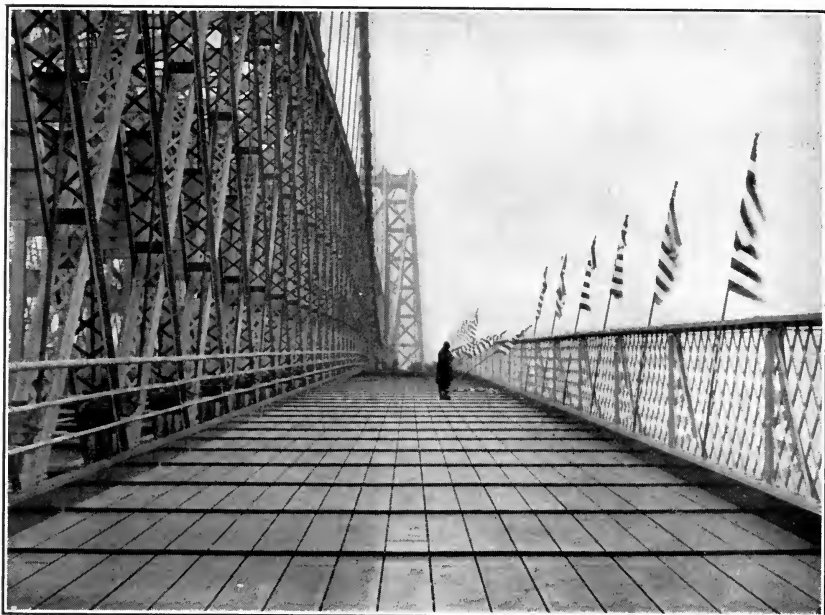
Steel underfloor (coated with Sabin Pipe Coating) ready to receive wood-block pavement, Williamsburg Bridge, N. Y. City.
