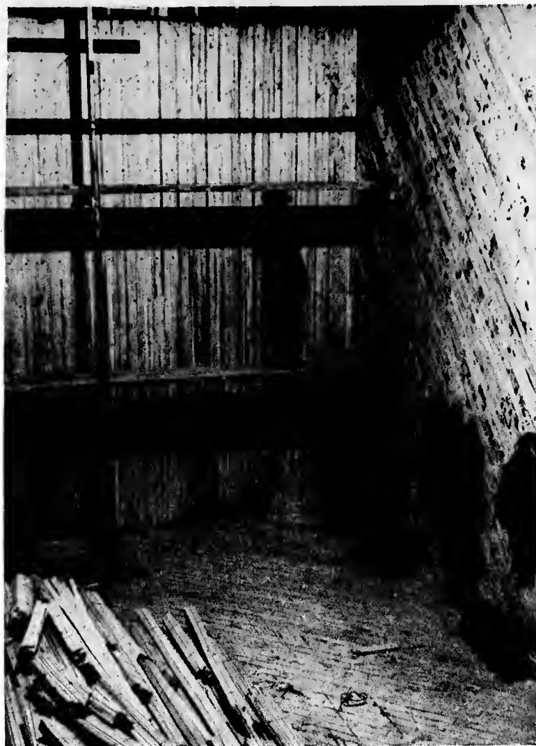
This picture shows the rear view of a court, built "like a bowling alley on end." The side walls and floor will eventually be covered with the maple lumber lying on the floor.
