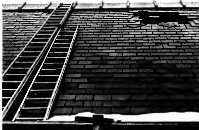
B & G estimates that damage to the Thompson Memorial Chapel in last week's wind storm will run $1500 for the slate, exclusive of labor costs. (Burghardt)
